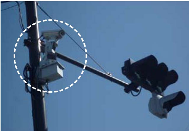
Equipment for preventing traffic accidents
